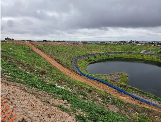
Plate 16. Frog fencing deployed around Offset Area 1 (Ecology and Heritage Partners Pty Ltd 30/08/2023).
