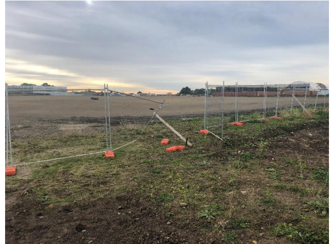
Plate 17. Safety fencing deployed around areas proposed to be constructed, with occasional gaps observed (Ecology and Heritage Partners Pty Ltd 03/07/2023).
